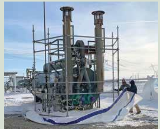
To prevent freezing of key power plant components, employees braved the cold to install wind screens.
